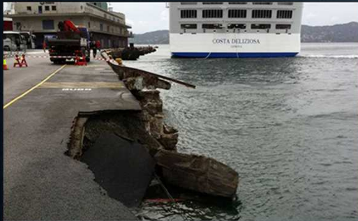
Cruise Ship Damages Quay
